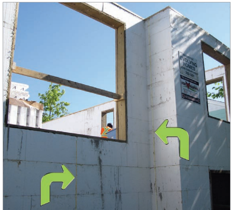
Here is a job, post concrete, that has been constructed exactly to the building dimension by properly stacking seams.
